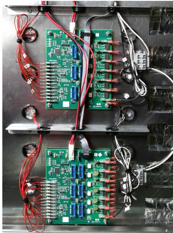
Fig. 7: Distribution board shown with display cables removed.
